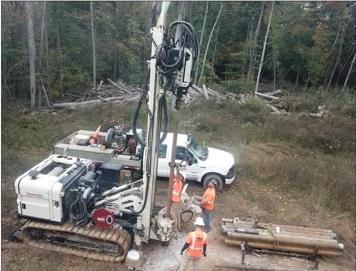
Figure 2: Drone view of sonic drill rig and crew at the Titan Project
