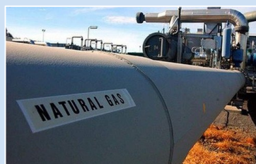
Natural Gas Pipeline
