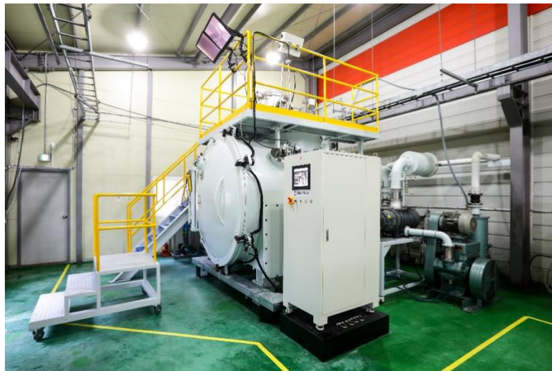
Figure 3: Ziron Tech Pilot Plant - Korea 2020
