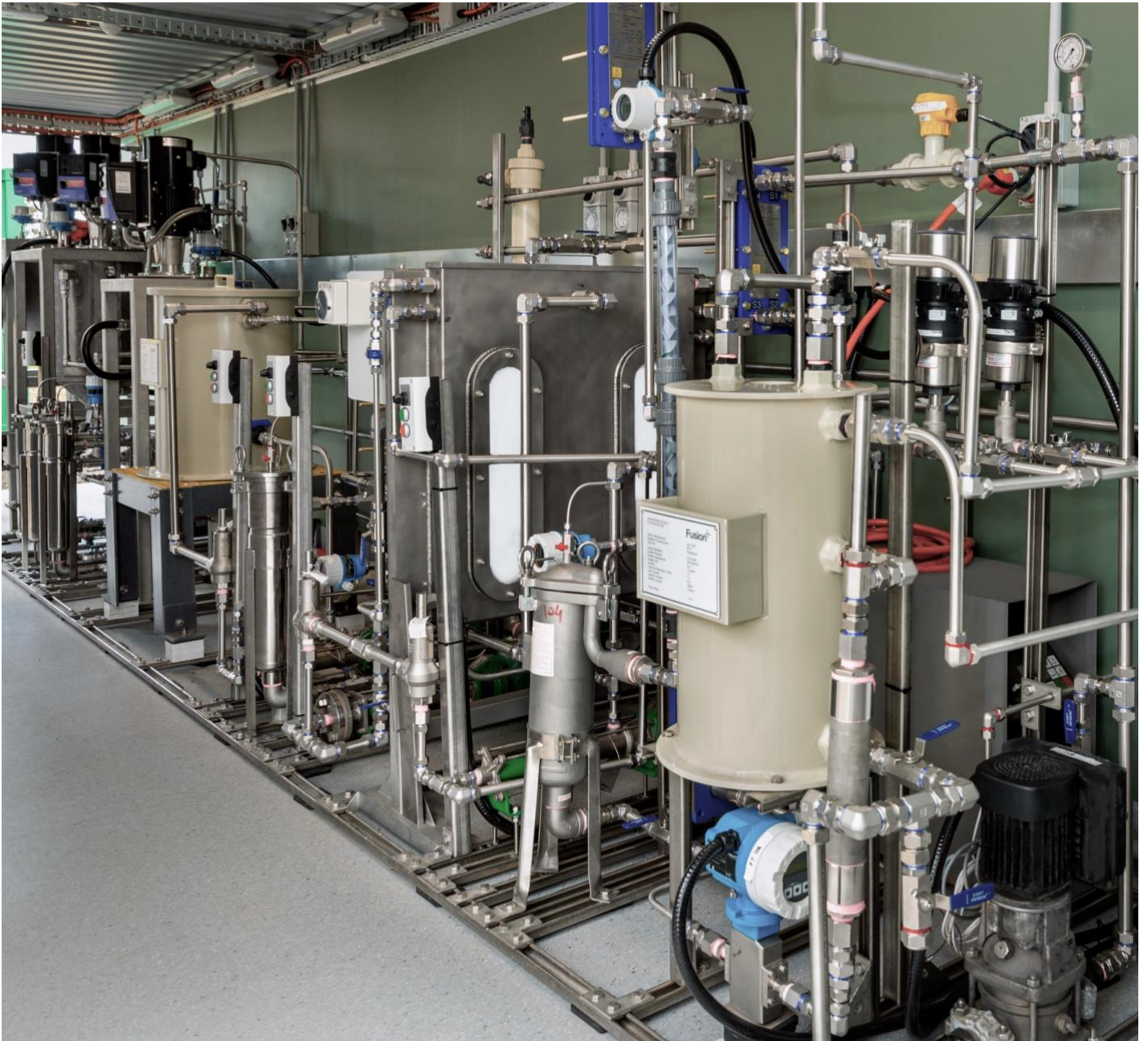
Recently installed state-of-the-art aMES™ pilot plant, currently undergoing pre-commissioning activities at Victoria University.
