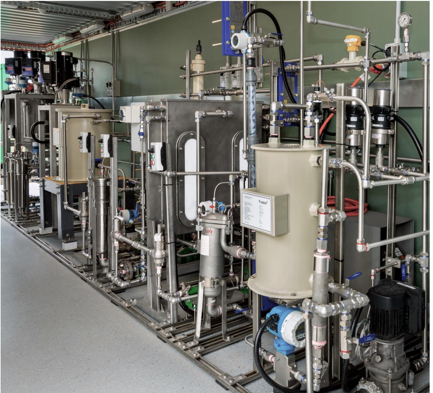
Recently installed state-of-the-art aMES™ pilot plant, currently undergoing pre-commissioning activities at Victoria University.
