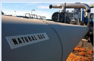
Natural Gas Pipeline
