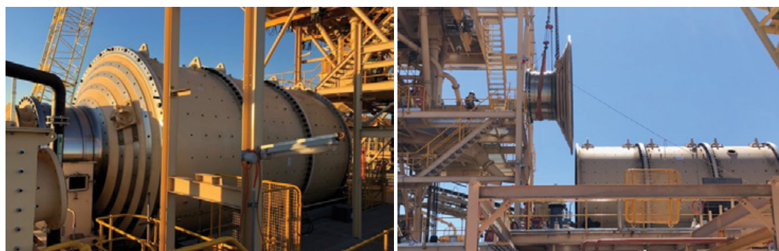
Figure 5.2: Installation of new ball mill as part of the CDO process plant expansion (completed)
