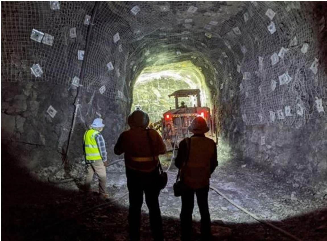
Figure 10: Development Jumbo at the decline face with traditional owners and senior wati members during a site consultation visit
