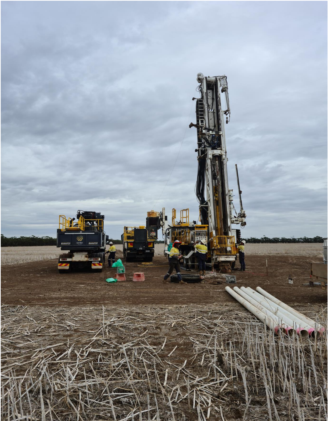
Figure 1 Strike Drilling collaring the first drill hole AWH001 today at West Wyalong
