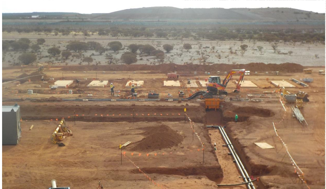
Figure 11: Concrete footings for 5x gas generator units and 2x additional footings for expansion activities
