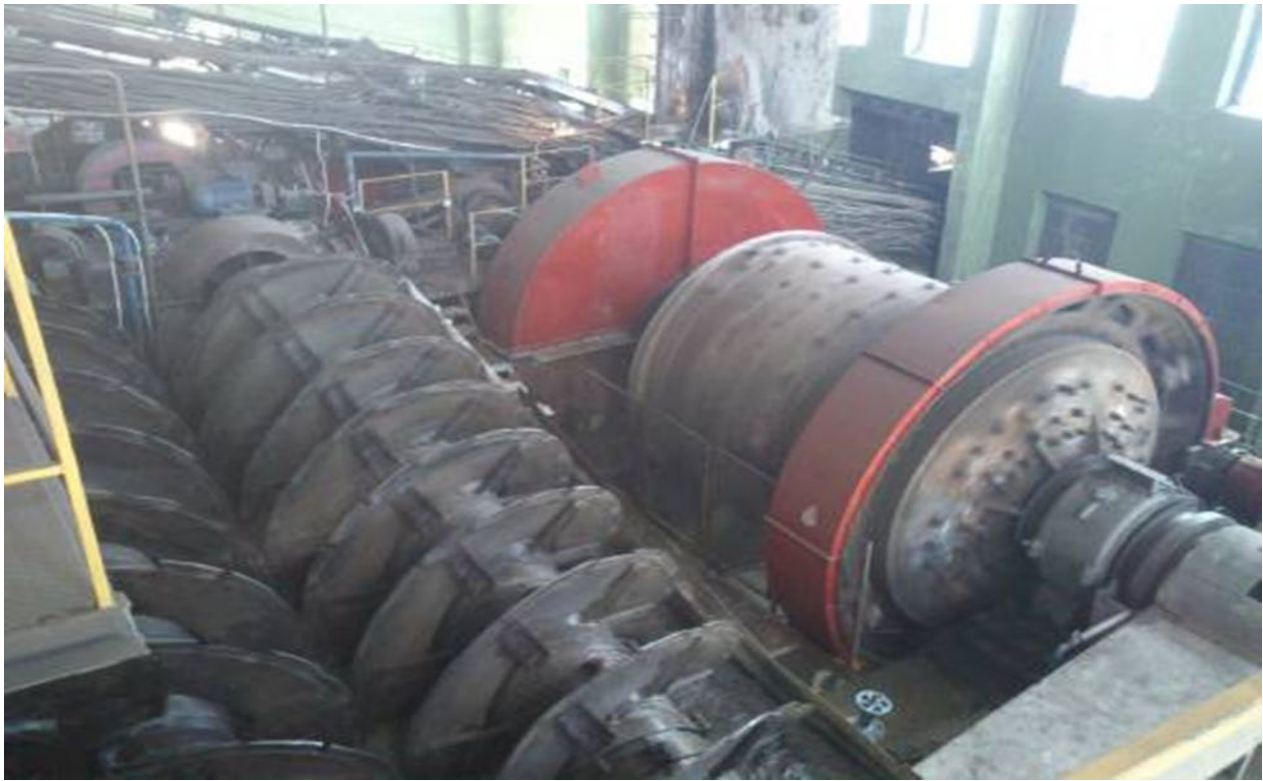
Zavaliievsky Graphite crushing circuit
