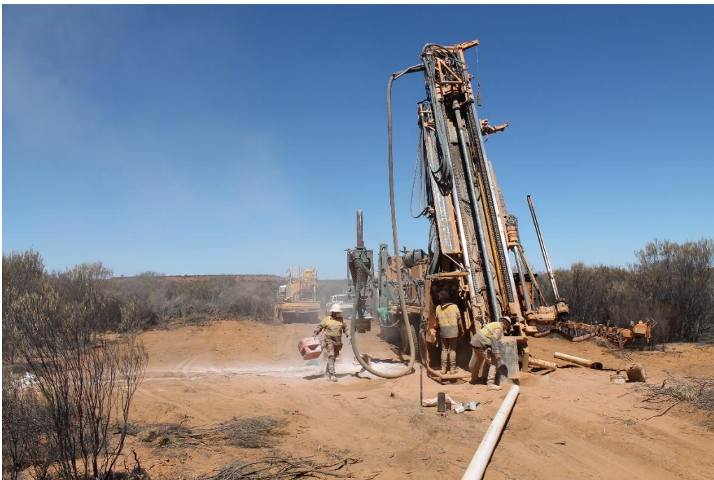
Figure 1: RC drilling at the Bonanza Gold Project with the Penny West waste dump in the background
