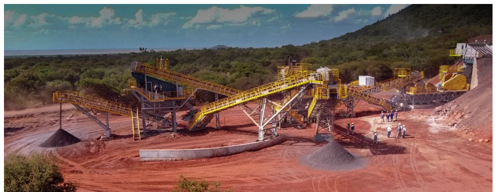
Figure 1: Tombador Project Crushing & Screening Plant
