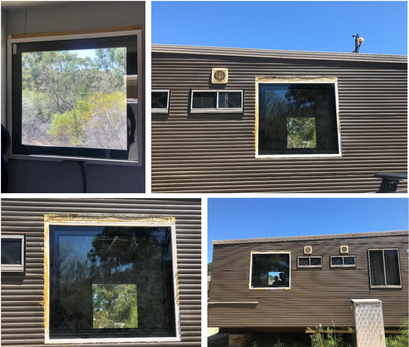
ATCO mining hut being retrofitted with ClearVue PV IGUs and Mirreco's Hemp panel insulation – view is through the installed IGU panels.
