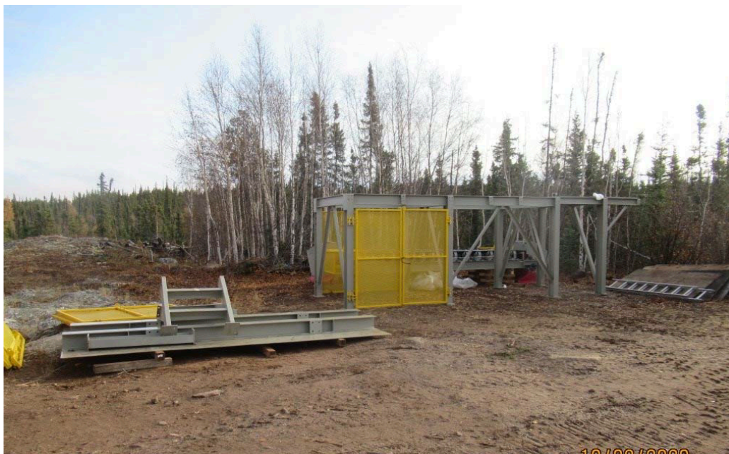
Figure 1: Ore sorter substructure for Vital Metal's Nechalacho rare earths project on-site and awaiting final placement
