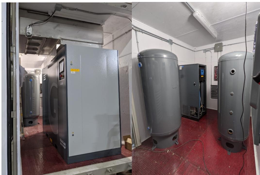
Figures 5: AC compressor (left) and receivers and dryer for Vital Metal's Nechalacho project are ready for delivery to site
