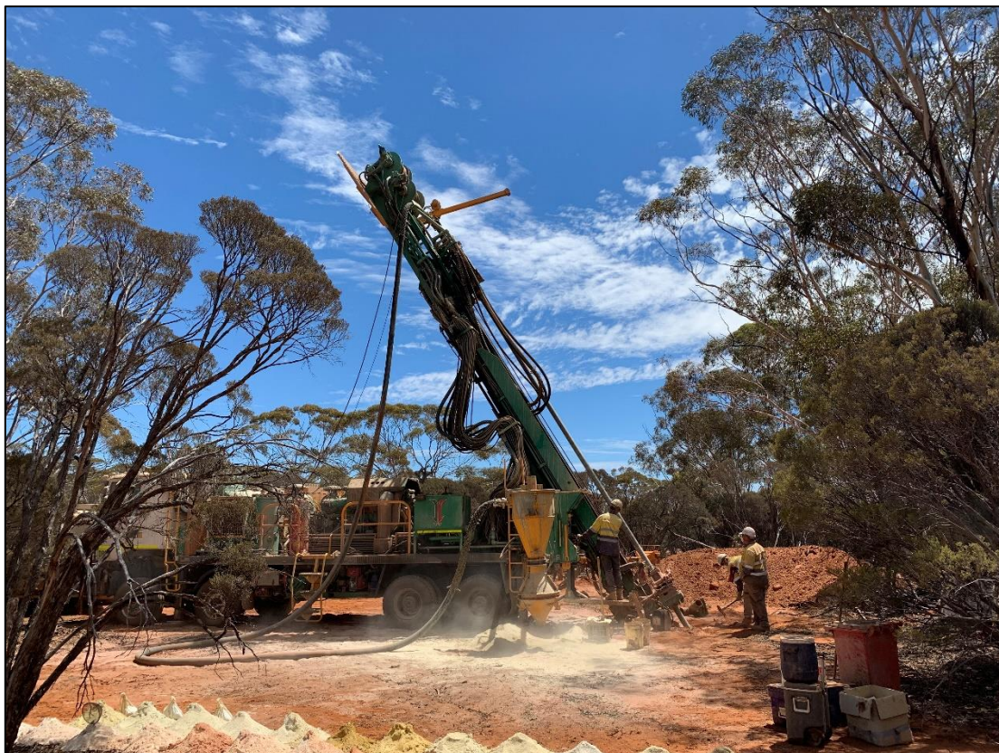
Photograph 1 –Seismic’s LMP 2000 multipurpose drill rig in action at the Nepean Nickel Project
