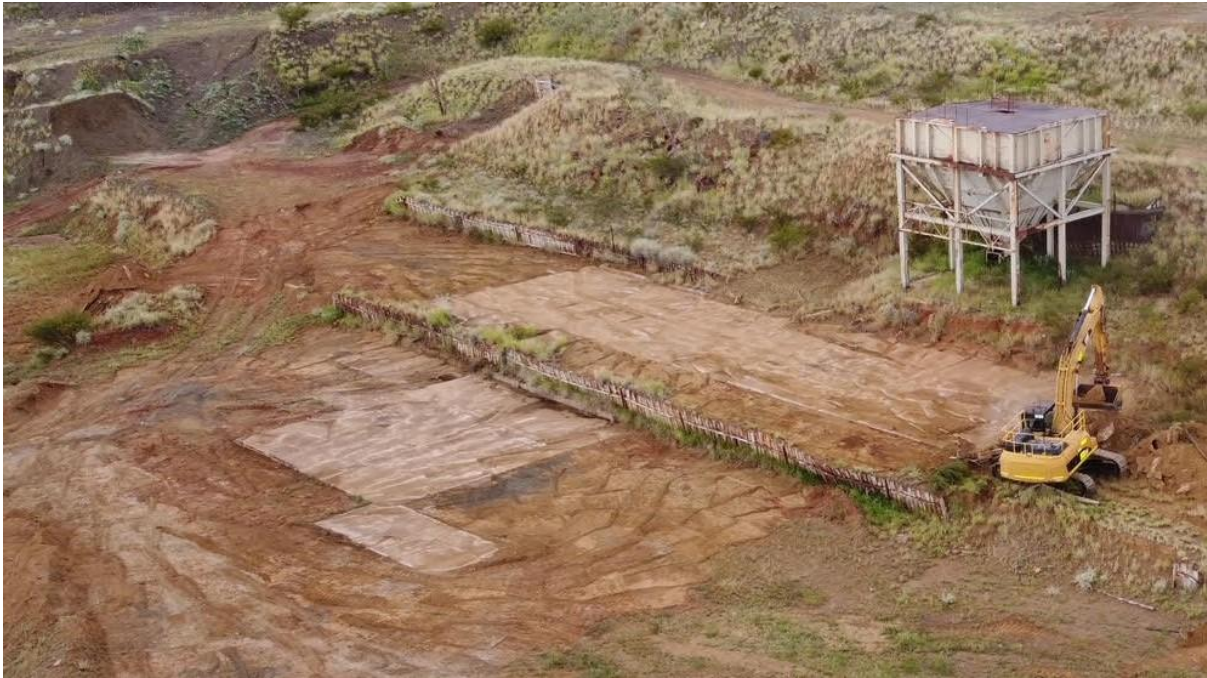
Figure 12: Exposing the original CIP concrete slabs, Mt Freda, next to Leach Vats Gold Processing.
