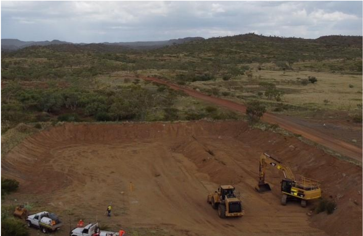
Figure 5: Unused 20,000 tonne empty Vat constructed by DMR in 1989 being detailed by Ausmex.
