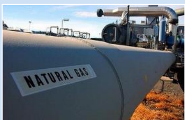
Natural Gas Pipeline
