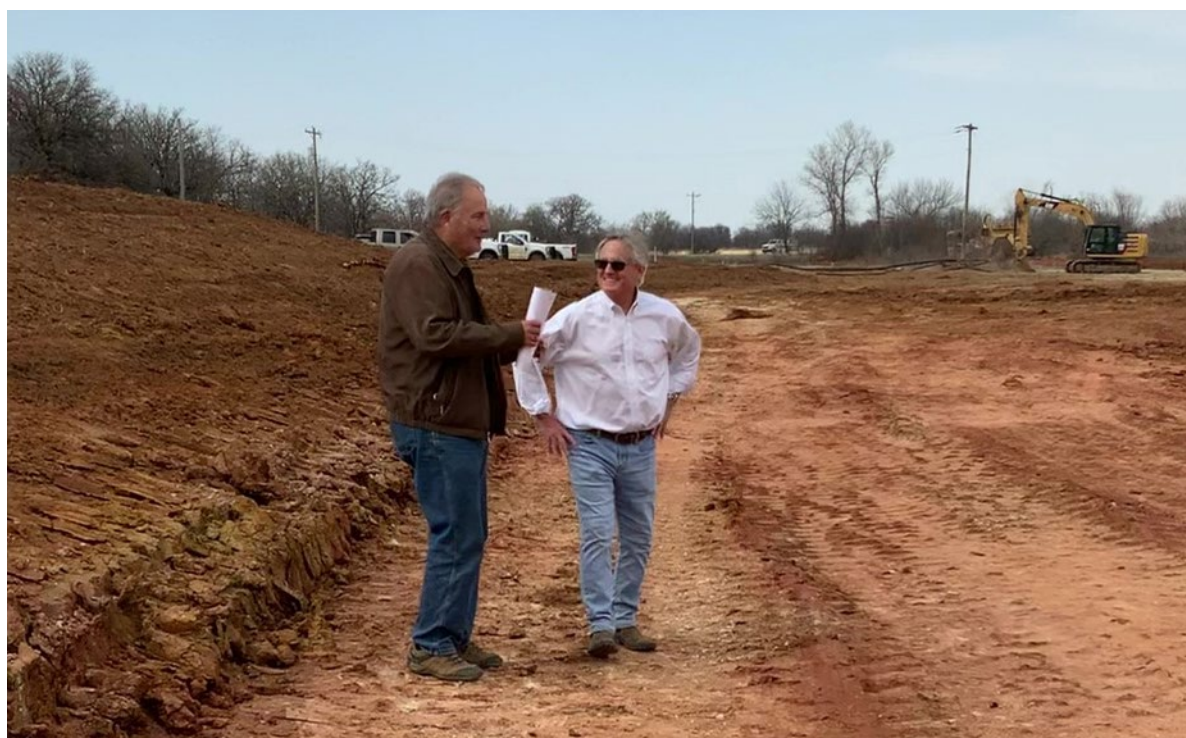
Figure 1. Black Mesa Energy President Chris Girouard and Vice President Operations, Lee Francis on site supervising Jewell Well drill pad construction
