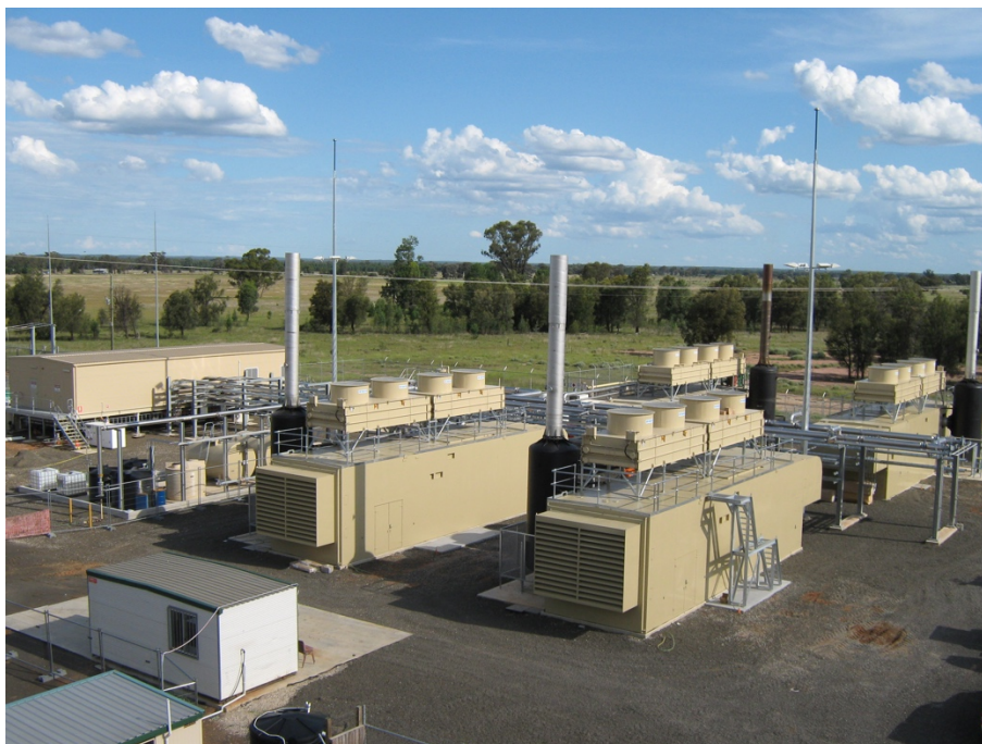
Wilga Park Power Station
