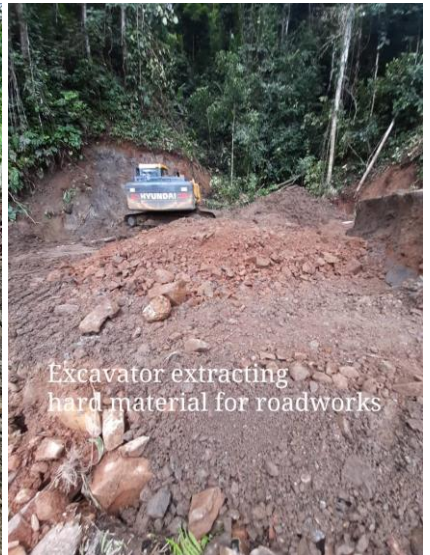
Hard material extracted from the road side ditch.
