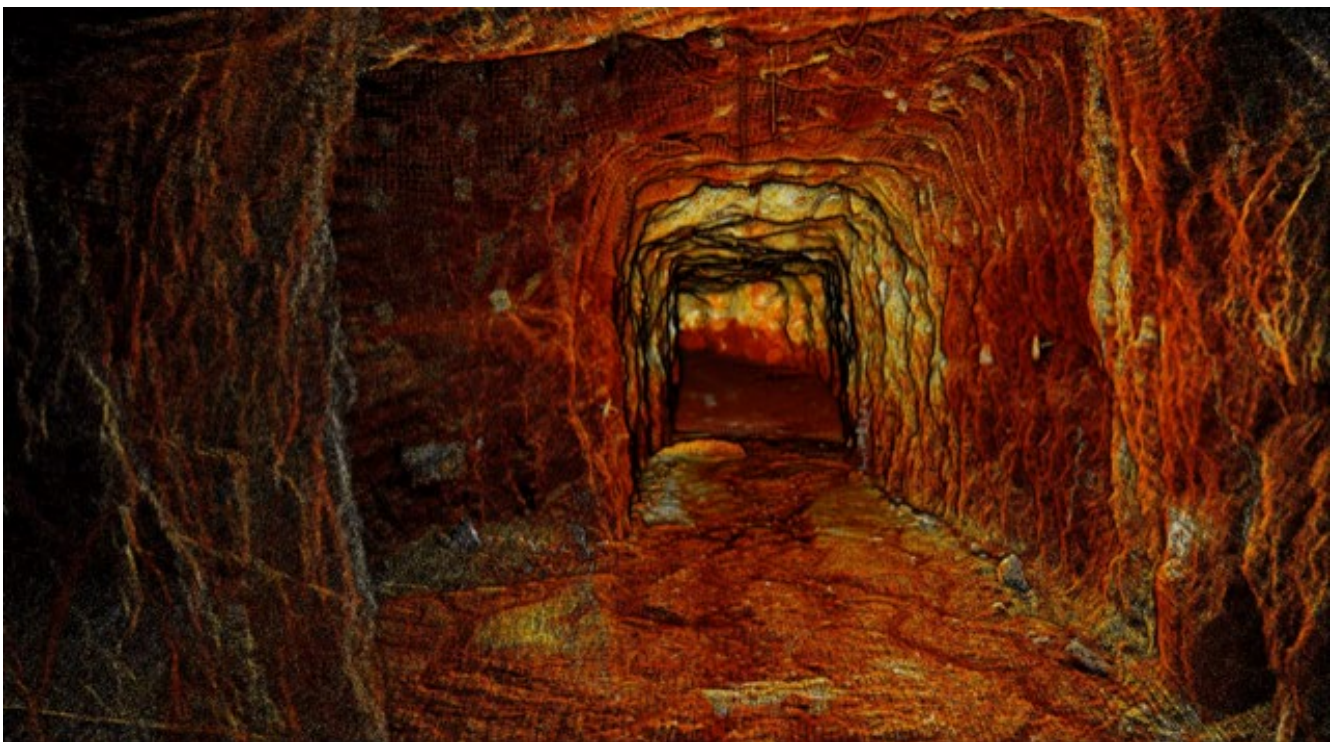
Figure 33; Processed image of First Hit Underground workings derived from Hovermap(R) LiDAR data.
