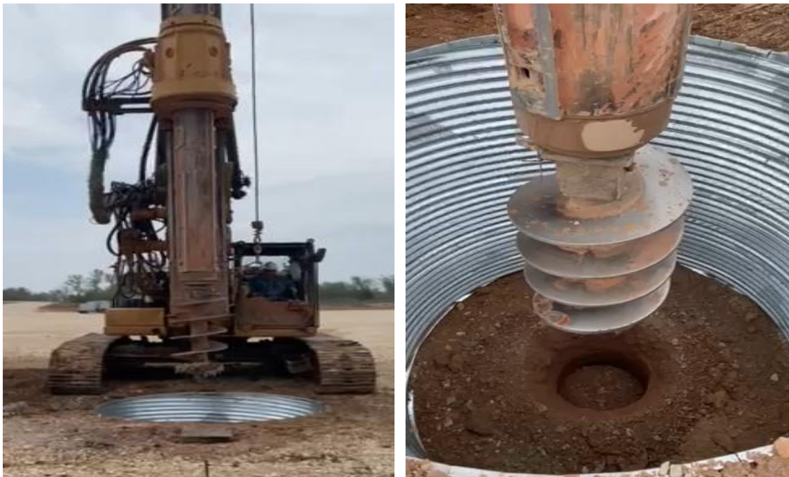
Figure 1. Drilling of the Jewell Well conductor casing hole using a specialised auger drill
