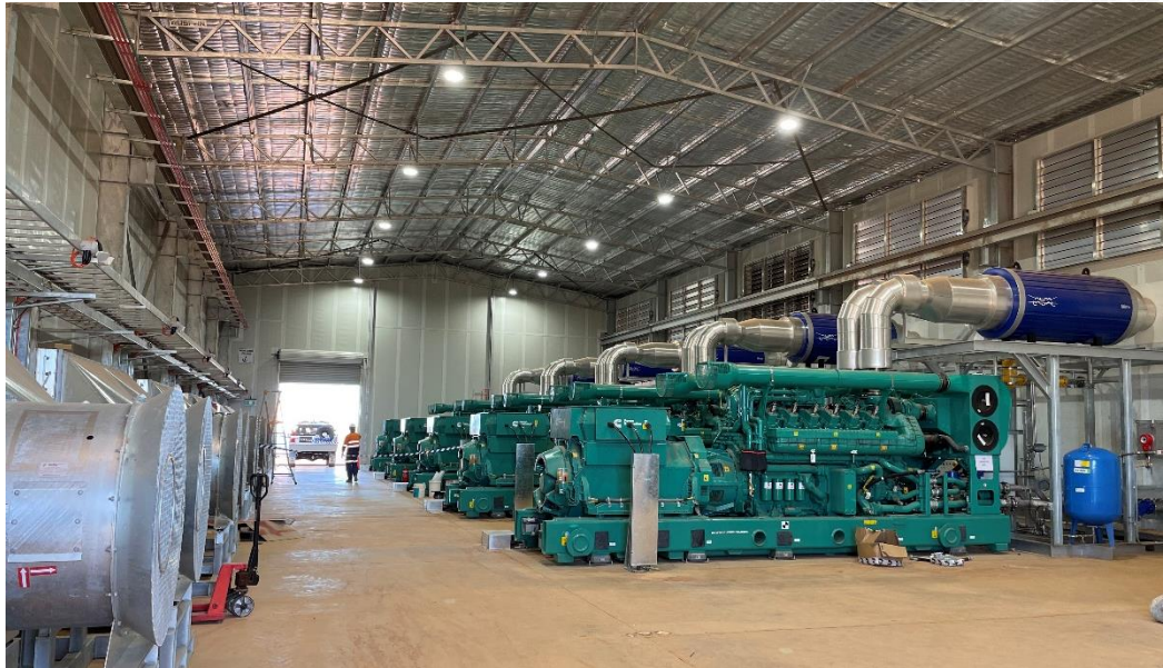
Figure 6: Five 2MW Cummins gas engines during commissioning
