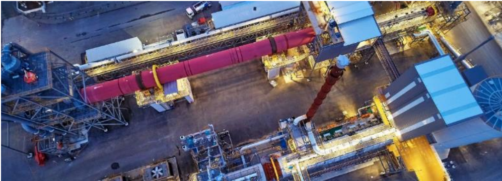
Above: Traditional spodumene gas fired rotary calciner
