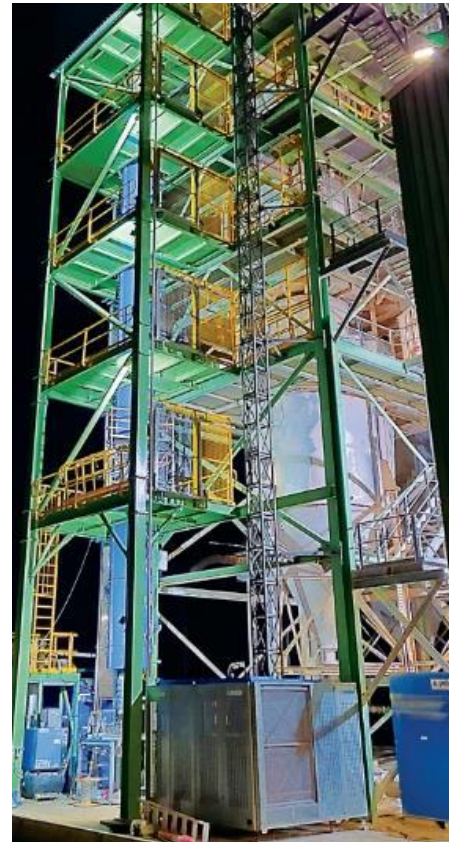
Left: Calix BATMn electric vertical reactor kiln enabling renewable energy powered calcination
