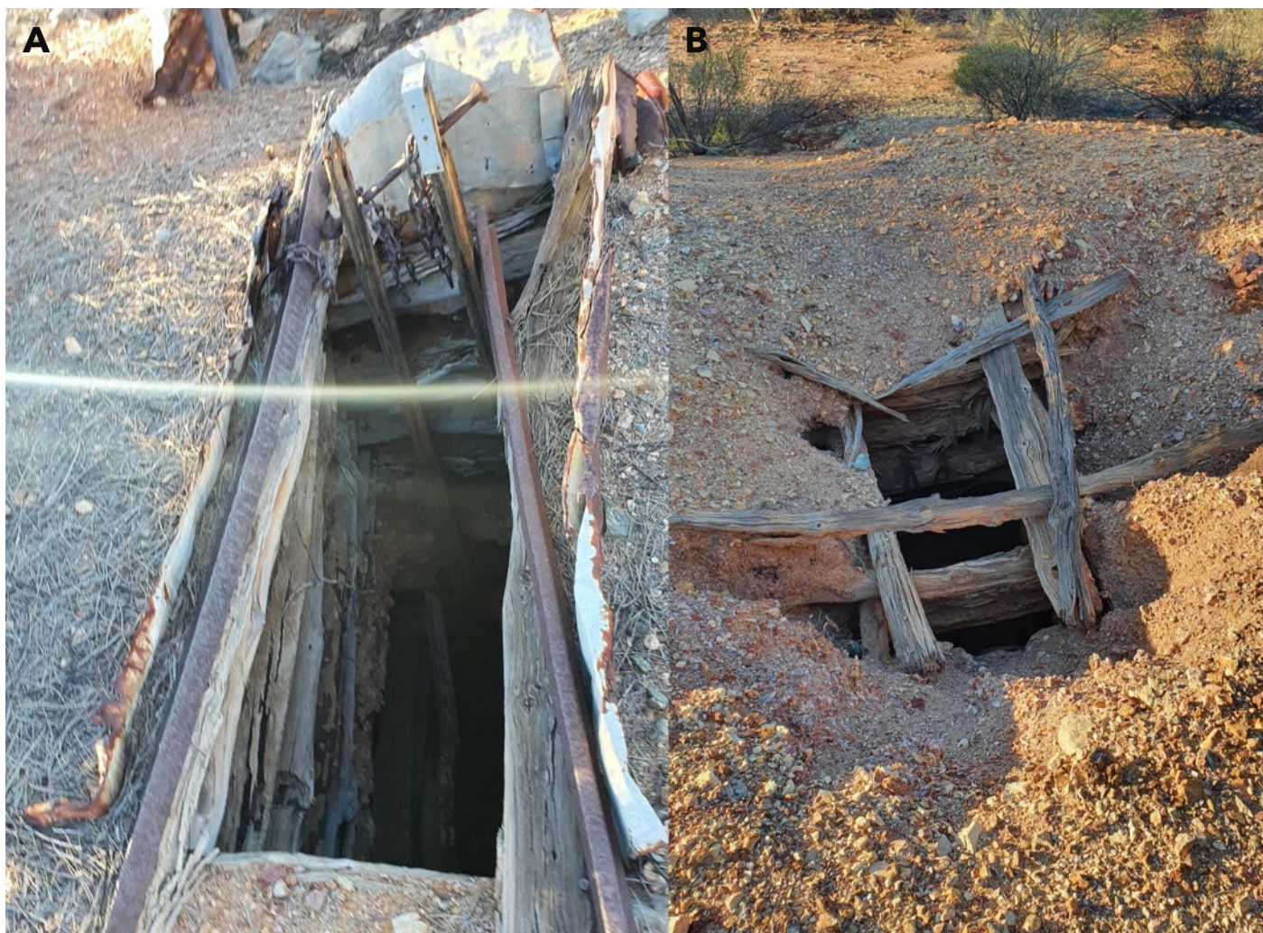
Figure 3; Two adjacent prospectors shafts located ~225m south of the surface expression of the First hit mineralisation. Image A shows the shaft which was scanned using the LiDAR system shown in Figure 4.
