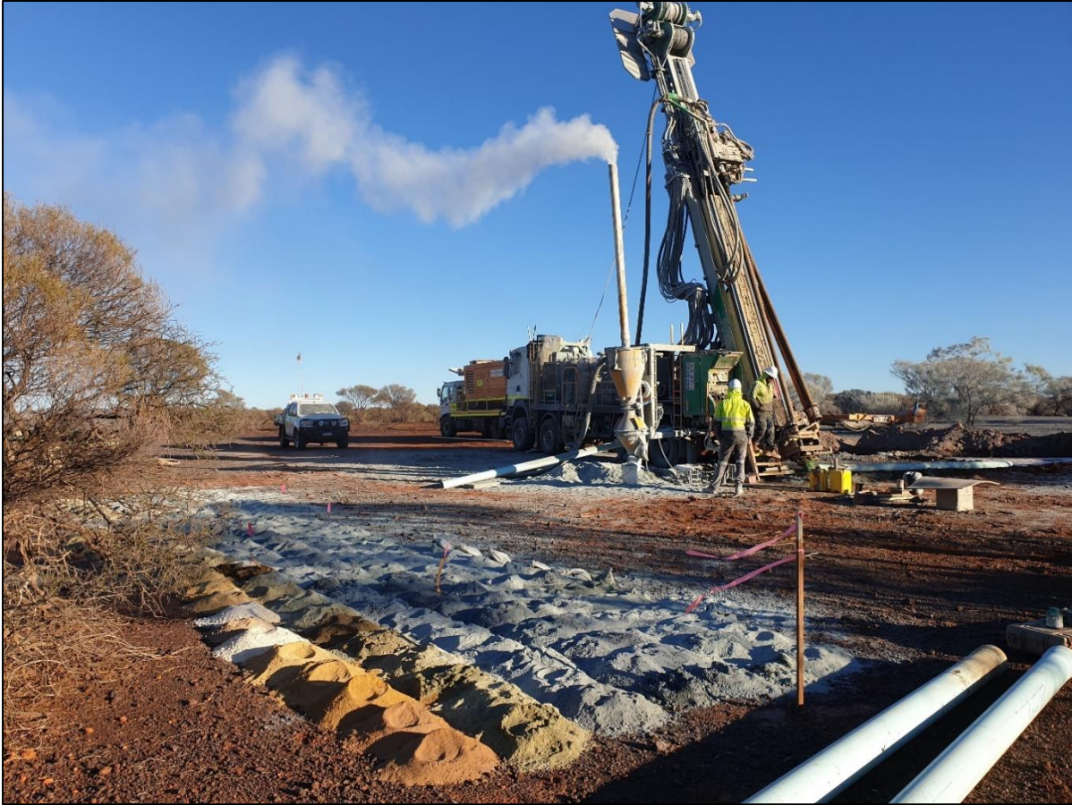
Photo 2 – RC drilling at the Firefly Prospect of the Leinster Nickel Project (drill-hole FFRC004)
