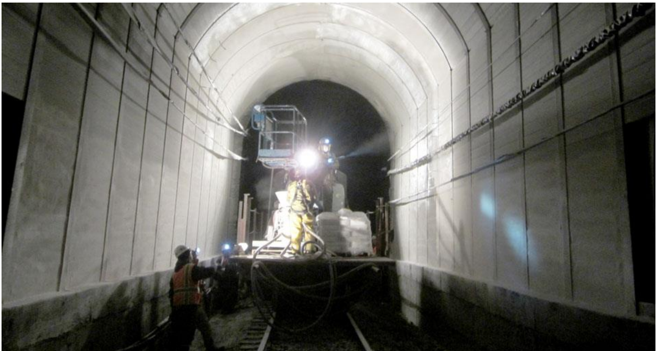
Figure 2. The interior of the Moffat Tunnel photographed during an earlier repair project (not involving EdenCrete®)
