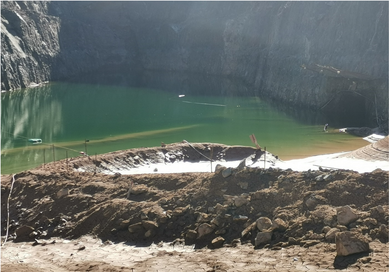
Caption | East Pit dewatering has exposed the second of three portal locations (Portal shown on right side of photo)
