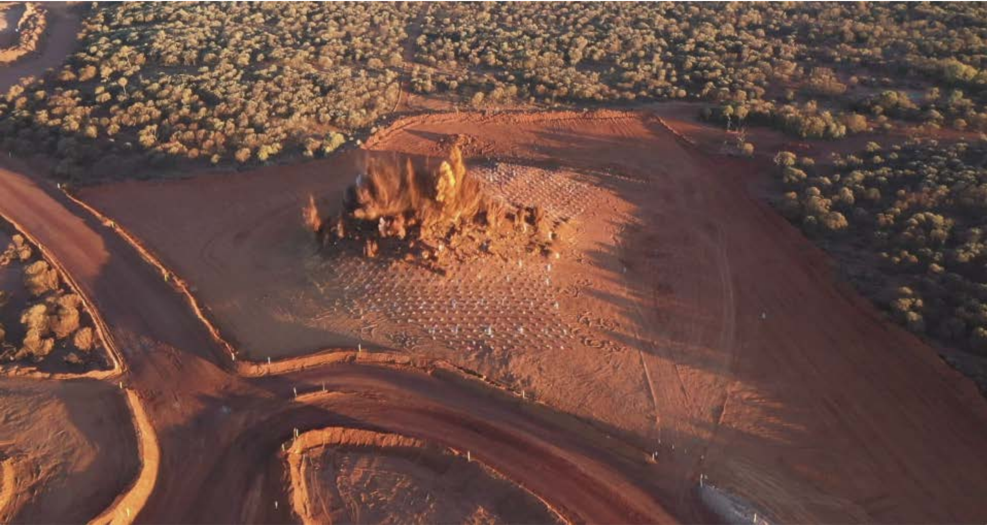
C4 Stage 2 – First Blast that occurred on 22 nd June 2021 at the South End of the Stage 2 Pit
