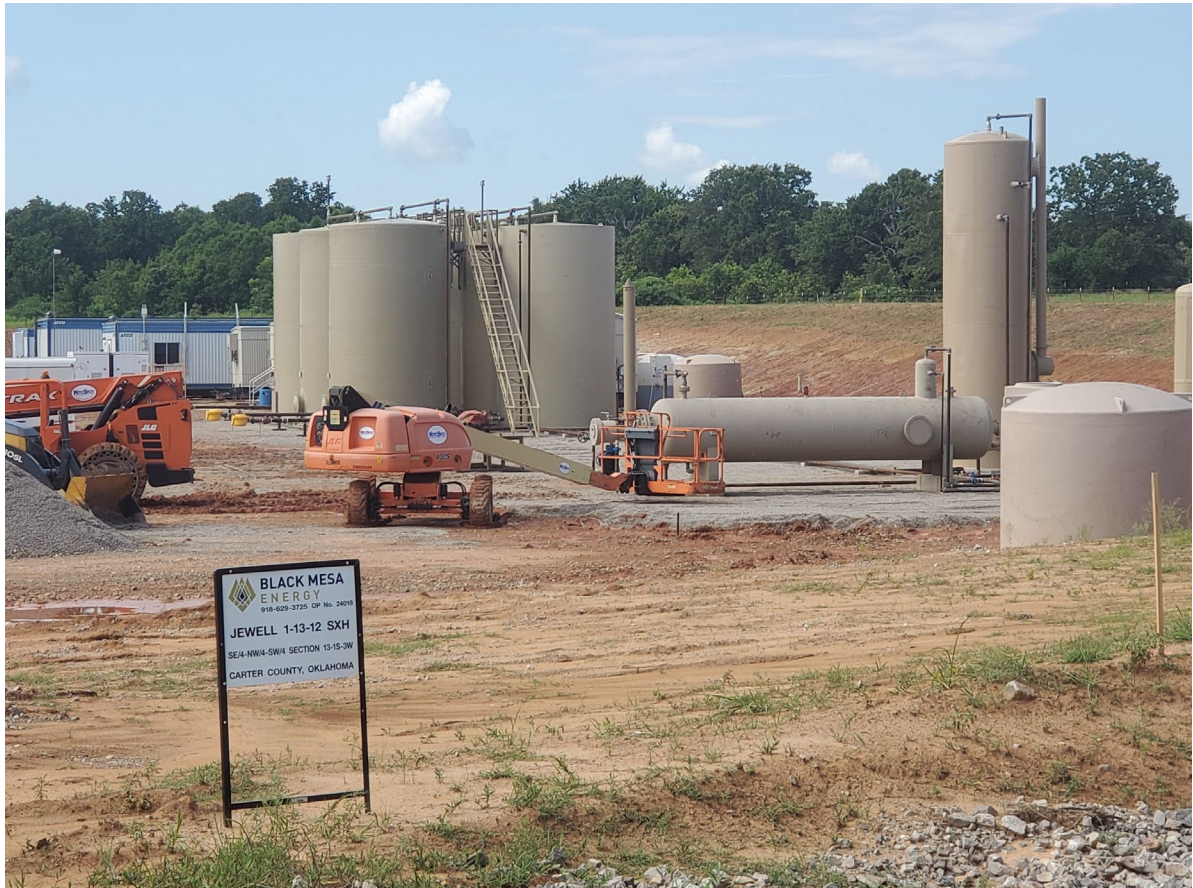
Figure 1: Jewell Well production facilities, tank battery (background) and separators (foreground).
