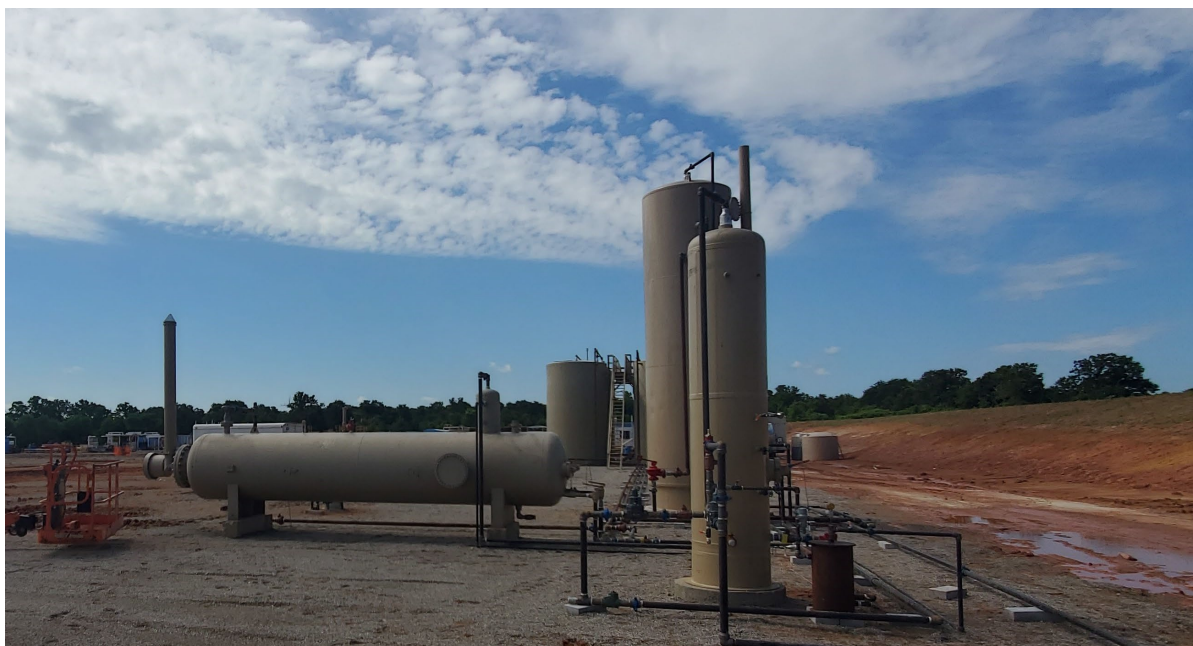
Figure 2: Jewell Well production facilities, close up with separators in the foreground.
