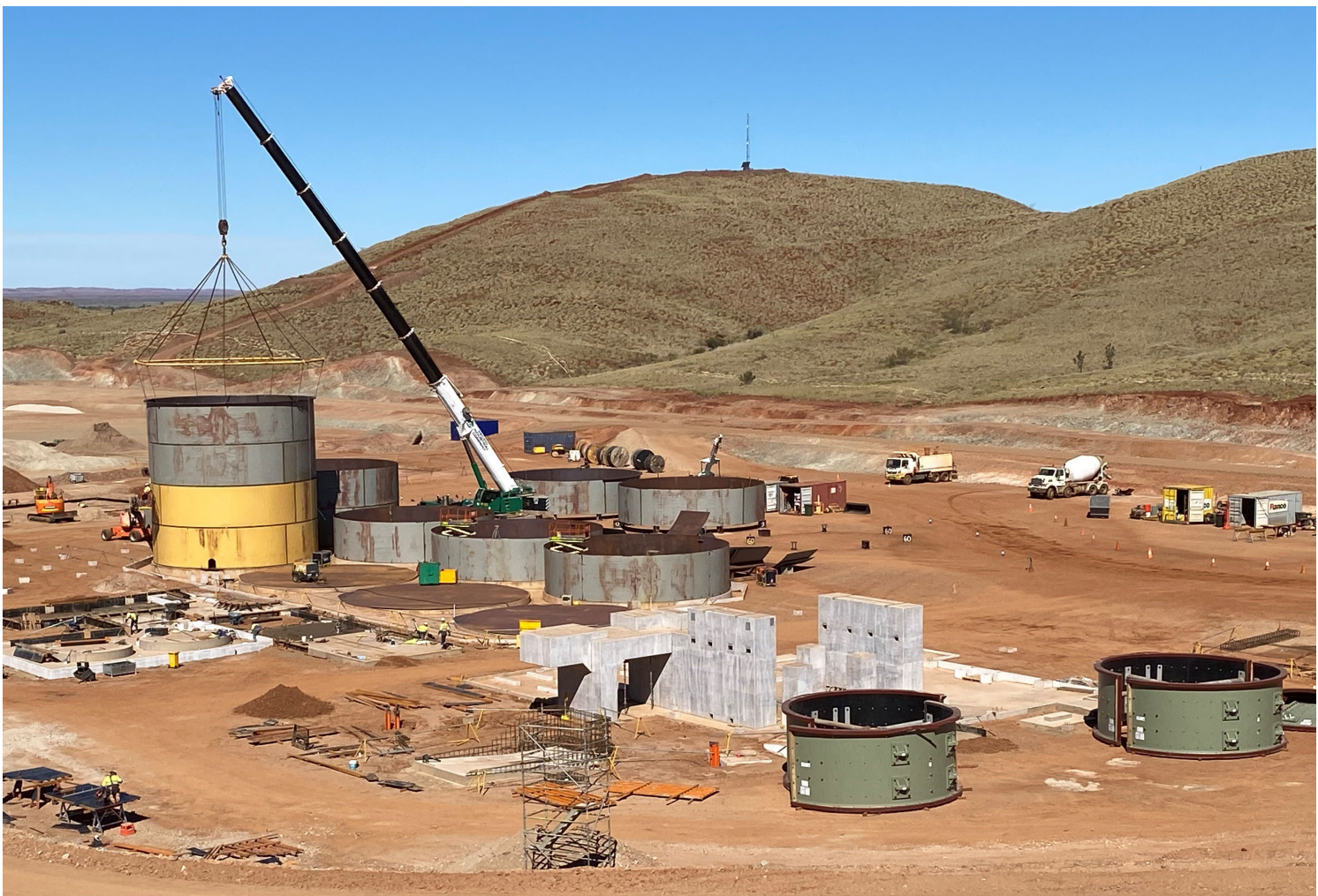
Figure 3: SAG Mill on Site
