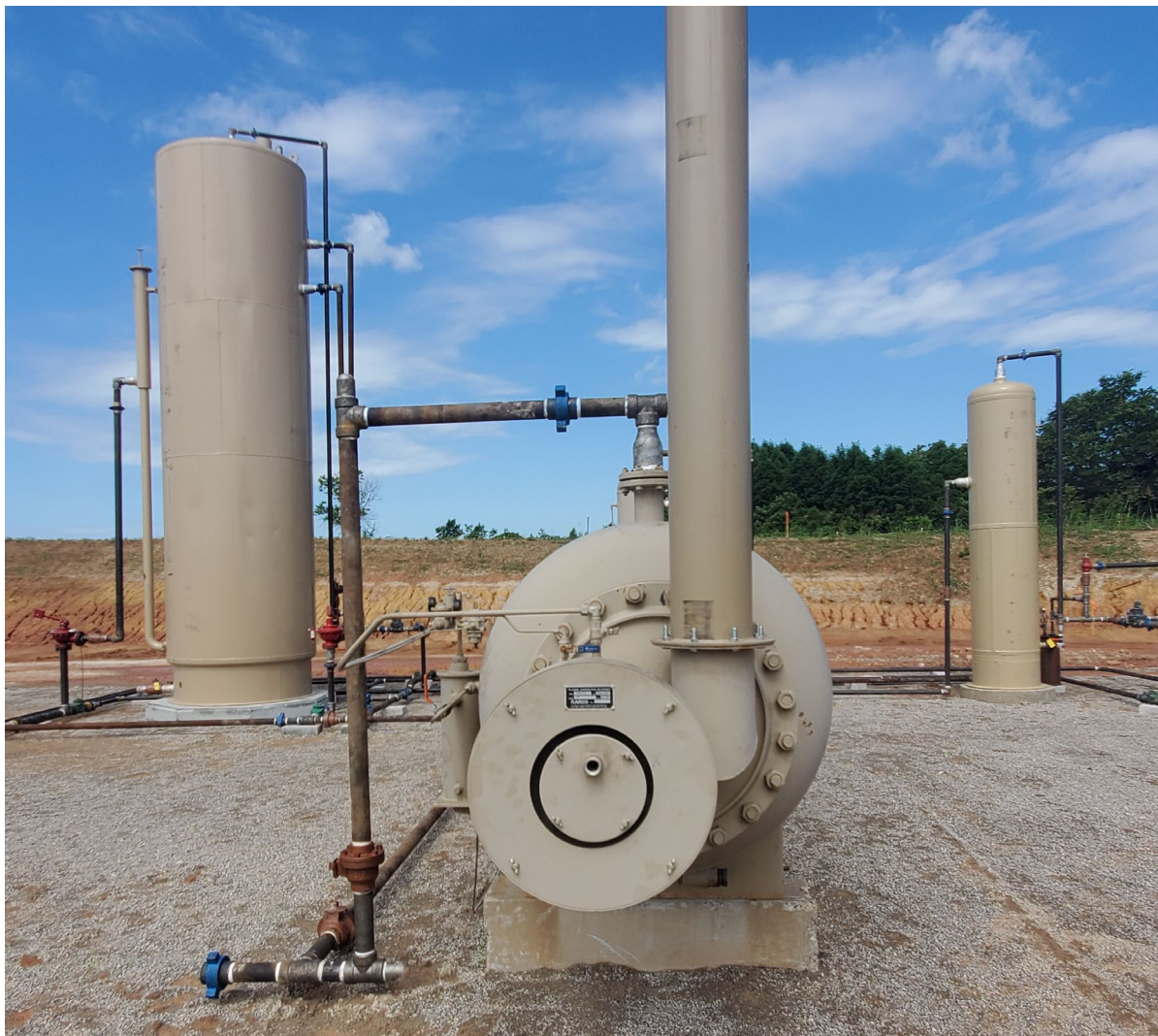
Figure 2: Separators set and plumbed-in on the Jewell Location in Carter County, Oklahoma
