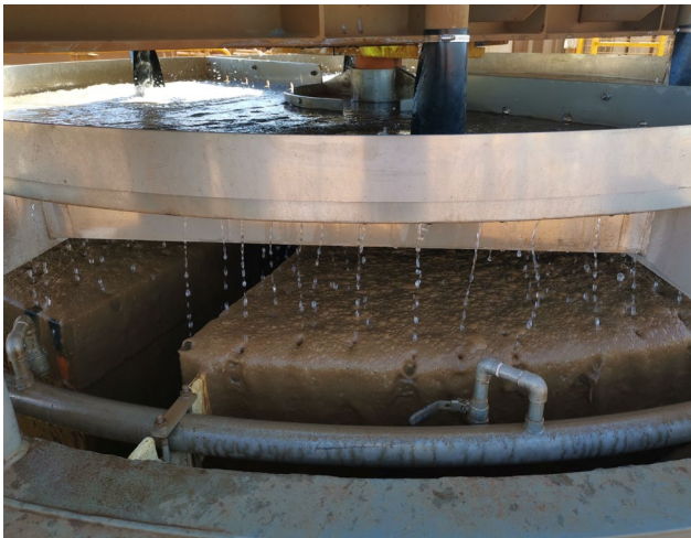
Commissioning of 2 nd Stack Cell
