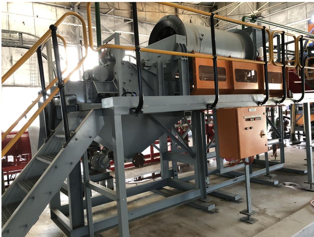
Figure 3: Scrubber and wet screen assembly at Bond Equipment, Johannesburg, South Africa
