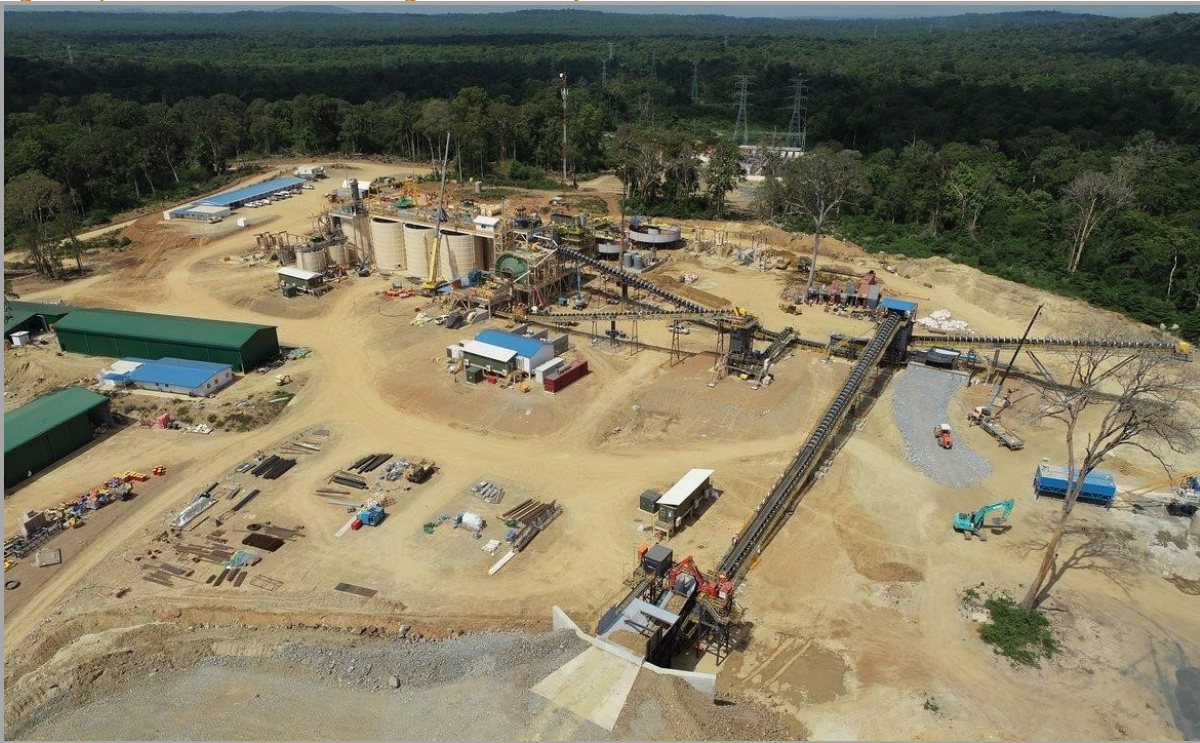
Figure 4 | Process Plant and Crushing Circuit - Complete and Commissioned
