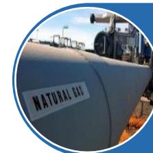
Natural gas pipeline
