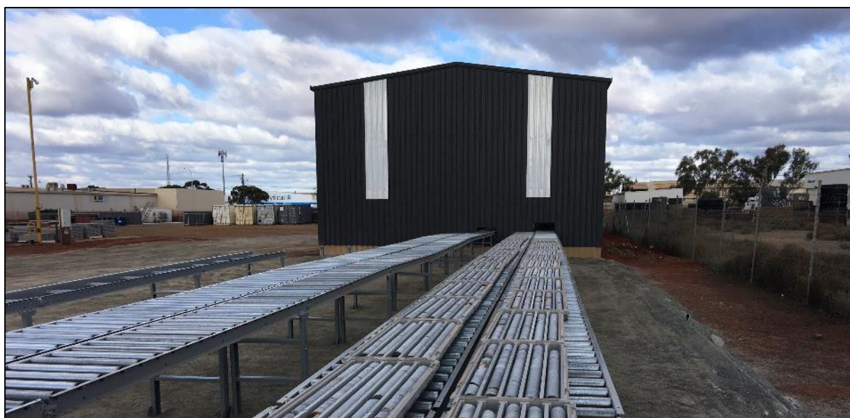
Figure 8: Roller racking at Iceni's Kalgoorlie core yard. The racks can hold 600m of NQ core which is fed to twin Almonte diamond core saws.
