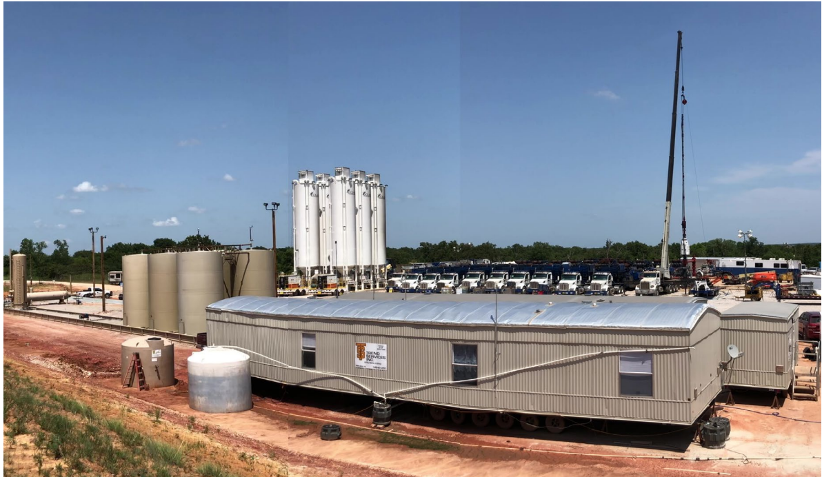
Figure 1: Panoramic view of completion equipment on the Jewell Well site, commencing multi-stage hydraulic stimulation.
