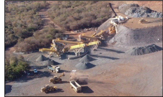
Crushing and Screening Plant
