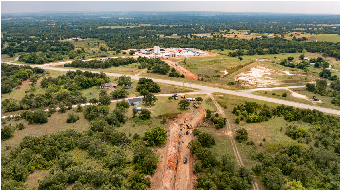
Figure 3: Gas pipeline construction from the Jewell Well site, under State Highway 7, to tie-in point at sales line.
