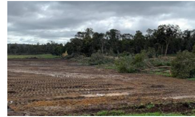
Great Eastern Highway Wooroloo Realignment Client: Main Roads WA Location: Wooroloo, WA Value: $8 million
