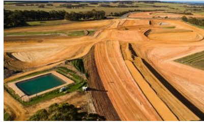
Albany Ring Road Phase 1 Client: Main Roads WA Location: Albany, WA Value: $55 million
