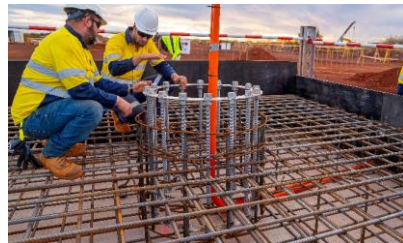
Mesa A and Mesa J NPI Works Client: Rio Tinto Location: Pilbara, WA Value: $39 million
