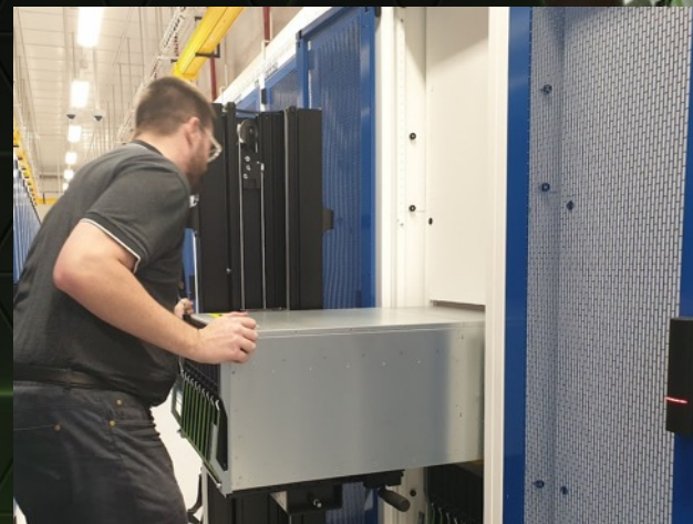
Photo: RTX server installation at NEXTDC P2 Perth.
