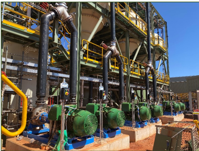
Flotation Circuit Pump Station
