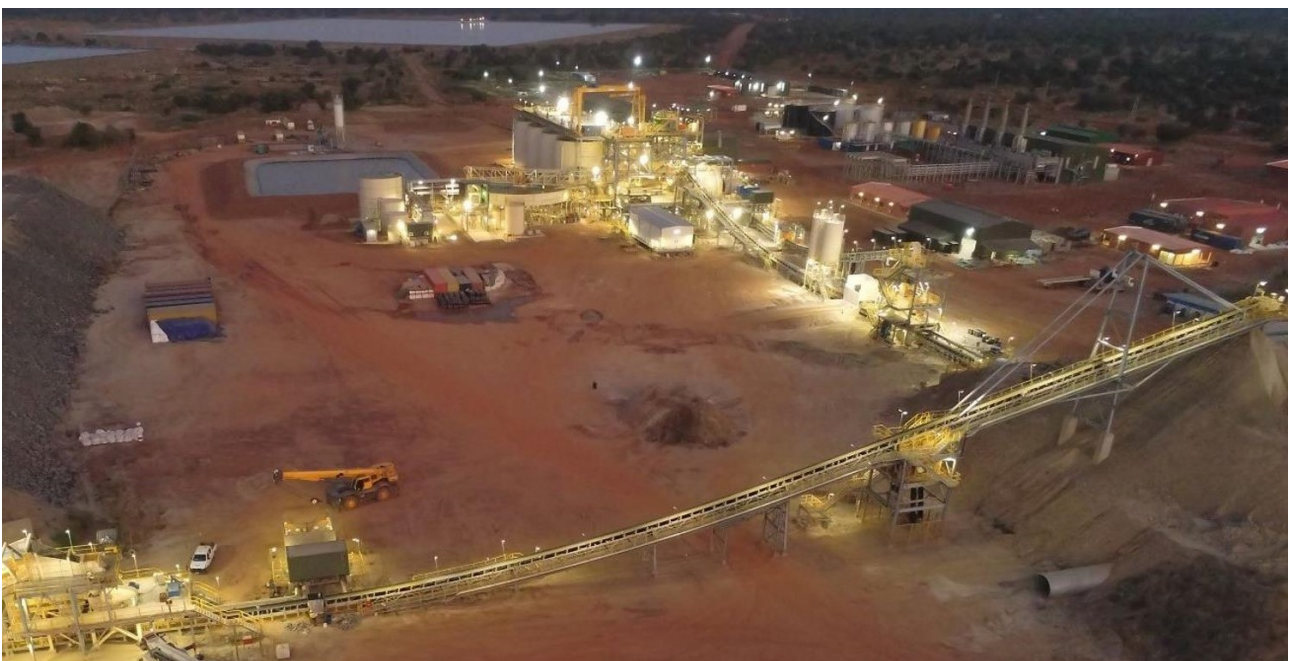
figure 4 – Sanbrado process plant
