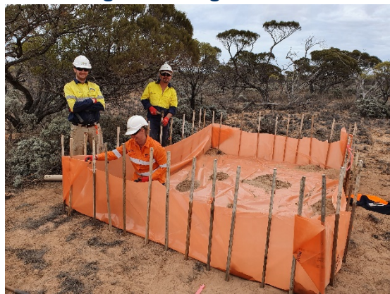
Above ground containment ponds used for drilling fluid capture
