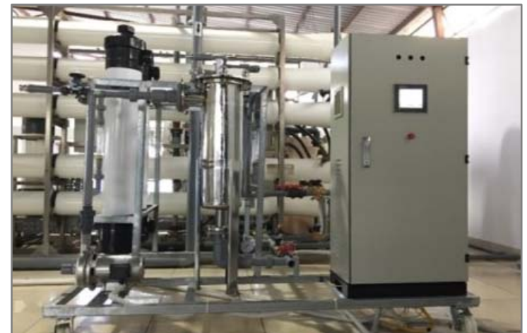
IMAGE: HF Nanofiltration membrane system deployed in Vietnam
