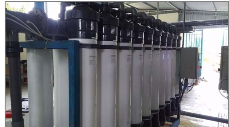
IMAGE: De.mem Ultrafiltration skid
