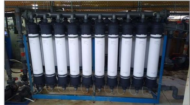
IMAGE: De.mem Ultrafiltration skid
