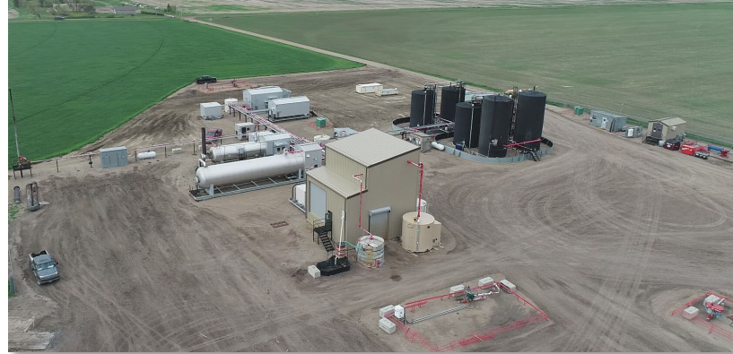
Bantry 2-29 Oil Battery and H 2 Sweet Plant
