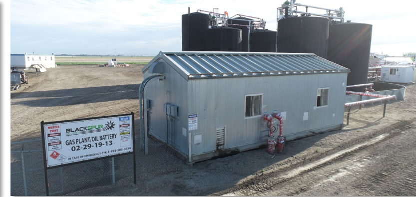
Bantry 2-29 Water Disposal Building and Tank Farm
