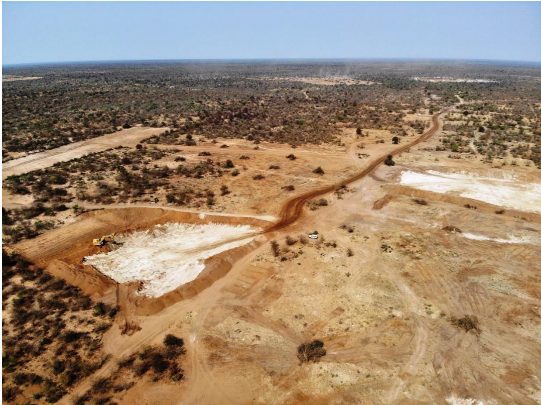
Figure 4: Clearing of topsoil T3 Stage 1 Open Pit and for the process plant and accommodation village in the background.
