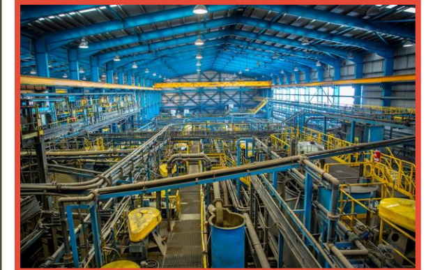
Central Processing Facility
