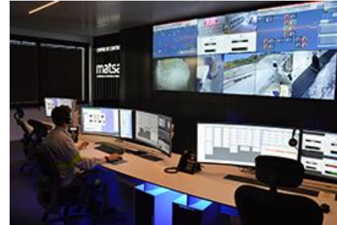
Centralised control room with digital technology and advanced emergency response hub
